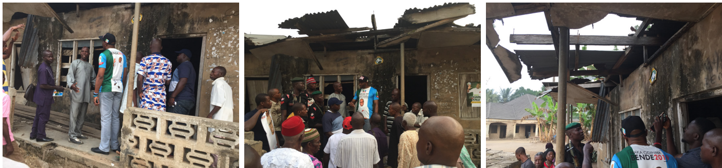
BEFORE - NTALAKWU HEALTH CENTRE (BEFORE REHABILITATION)
