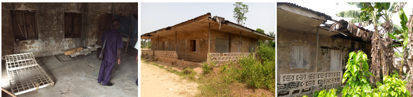
BEFORE - NTALAKWU HEALTH CENTRE (BEFORE REHABILITATION)
